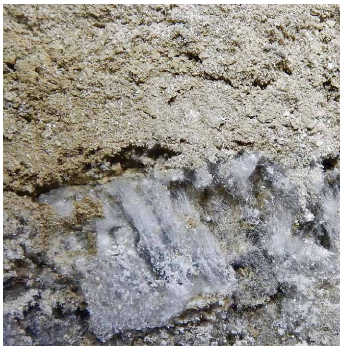
Figure 20. Mixed sulfates on passage wall.
