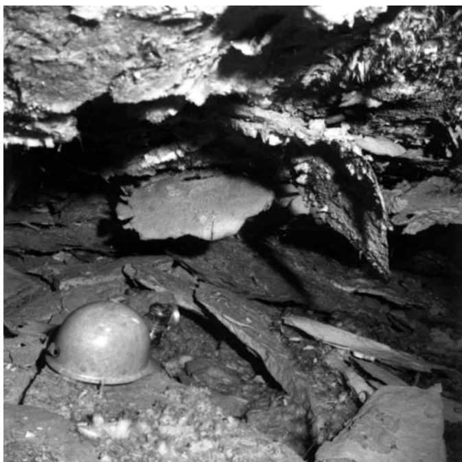
Figure 3. Thin plates and other fragments, some held to the ceiling by gypsum, in Upper Turner Avenue (Type II breakdown). Hardhat provides scale.
