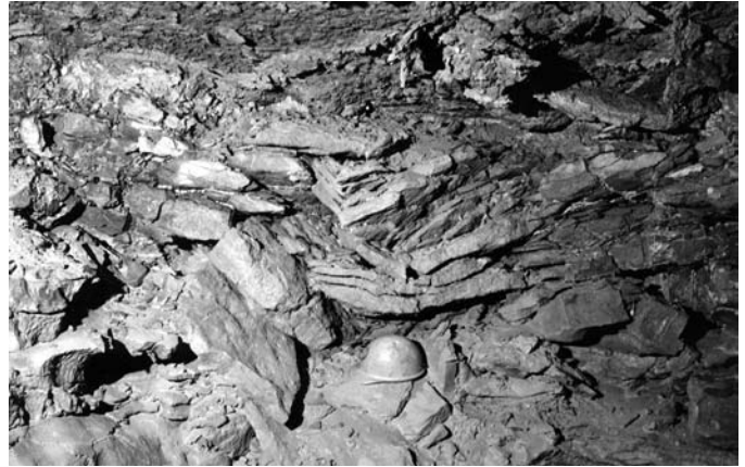
Figure 1. Rubble wall caused by gypsum deposition along bedding planes. Note hardhat for scale.
