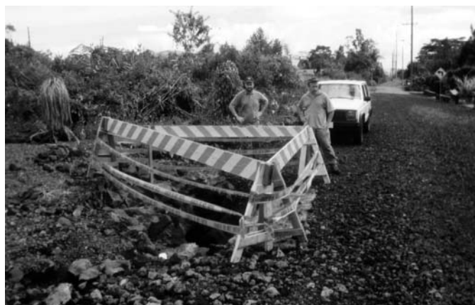
Figure 9. January 2001 photograph of overflow point of Kaumana Cave, in Kaumana community resulting from November 2000 flood. The location is the site of a former opening of the cave which was bridged to permit road construction.
